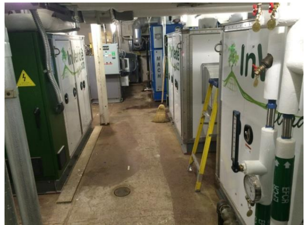
Three InVerde CHP Units at Intrepid
